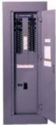
Figure 22: Panelboard (flush wall-mounted).
