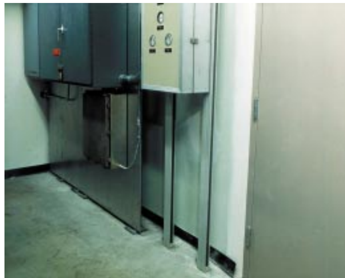
Figure 155: Two different ways to support control panels: using a metal plate attached to floor and ceiling with steel angles (left); using struts extending to floor and ceiling (right).
