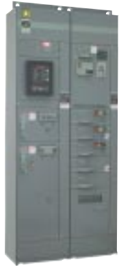
Figure 38: Low voltage motor control center (floor-mounted).
