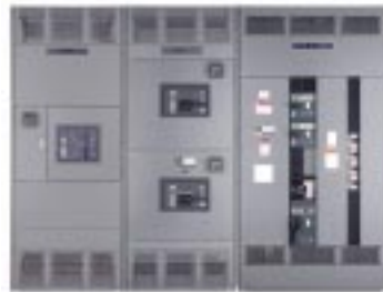
Figure 27: Low voltage switchboard (floor-mounted).
