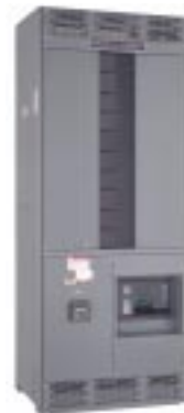
Figure 28: Low voltage switchboard (floor-mounted).
