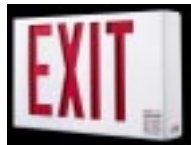
Figure 13: Exit light/lighted signs.
